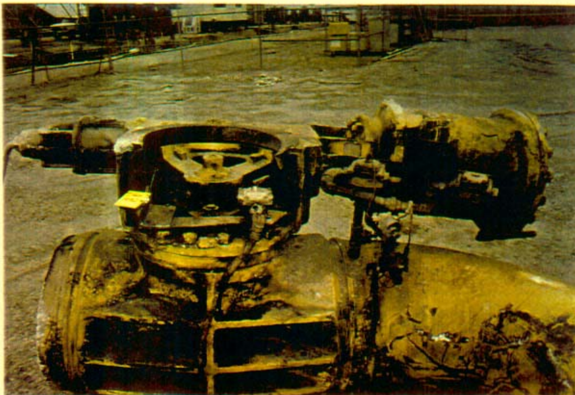
5-FG-24 Main Gas Trip Valve
