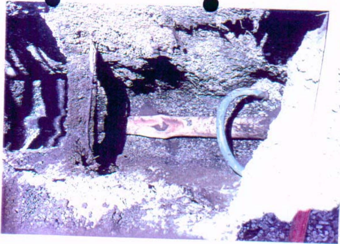
Collapsed section of sanitary sewer pipe was located in Area #4 on Drawing KCPL-8 under Tab 15.
