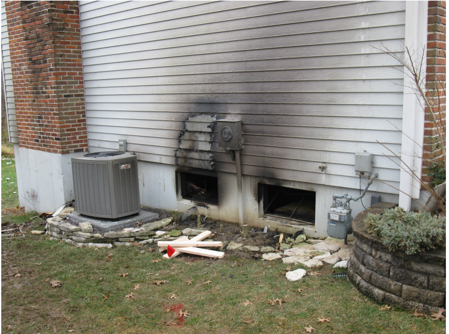
Photograph #14-- Showing damage at left front side (location of gas meter) of 5730 Mango Drive (Photograph taken by Staff).
