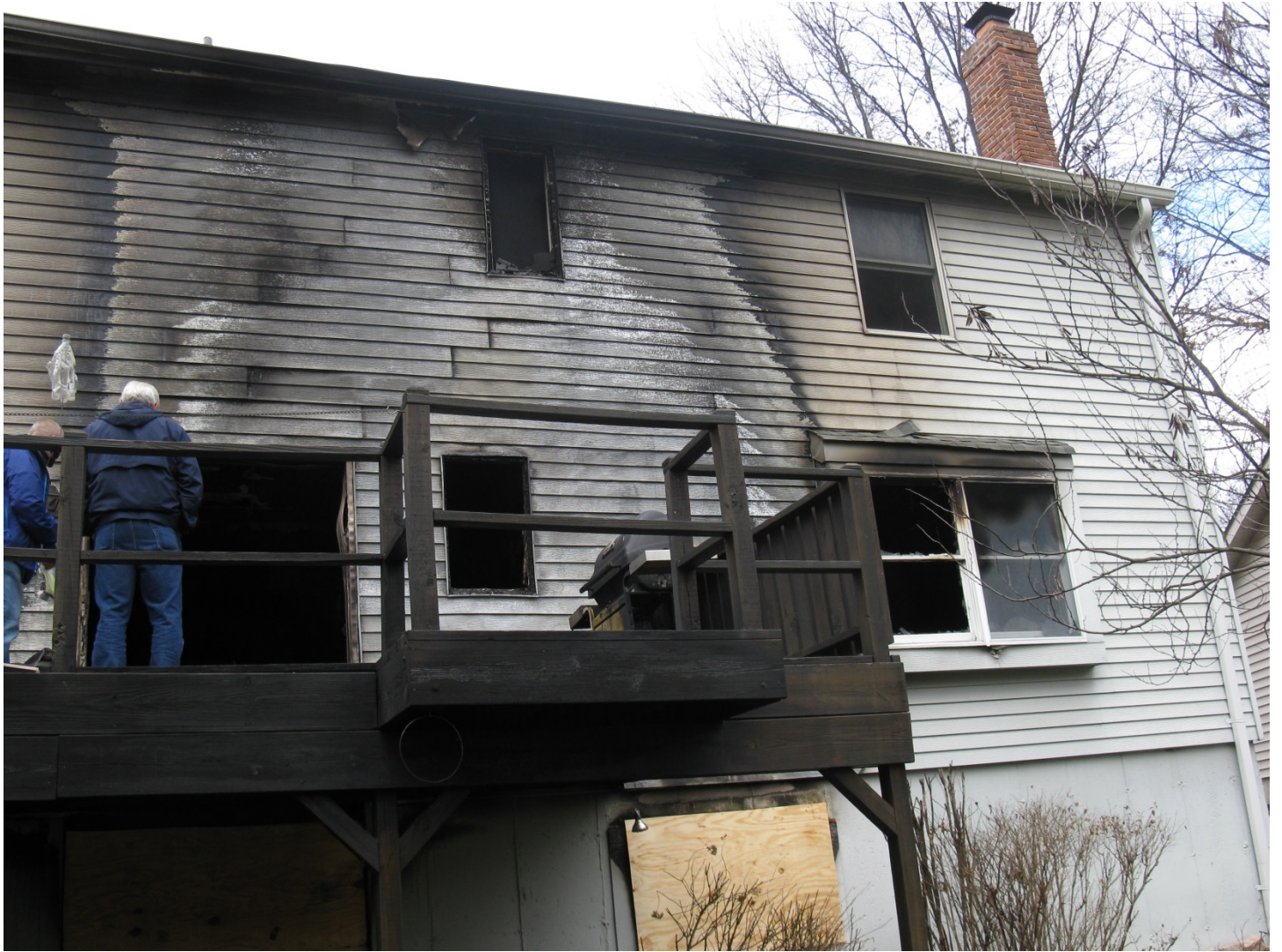
Photograph #15—Showing damage to back side of 5730 Mango Drive (Photograph taken by Staff).
