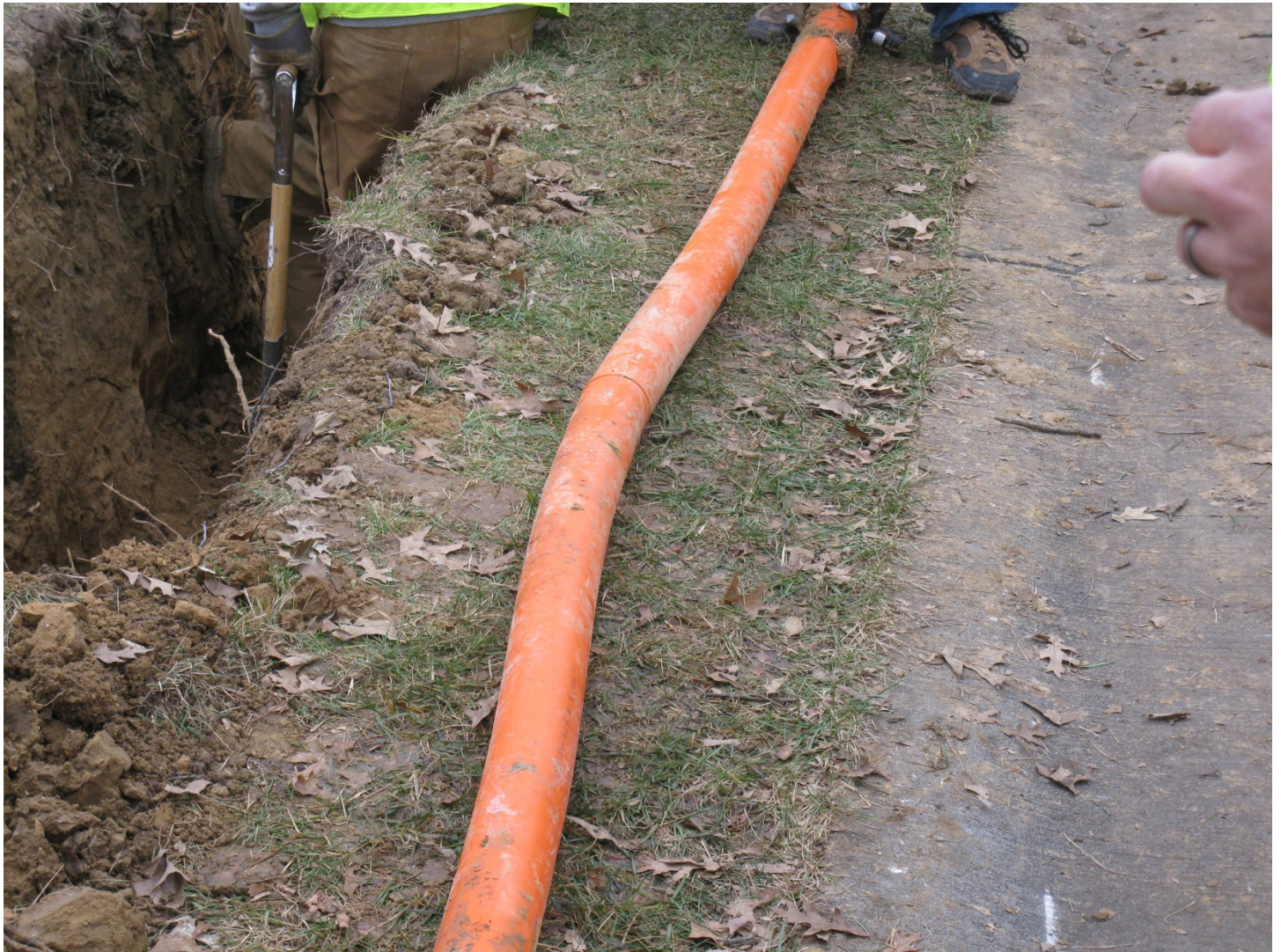
Photograph #19– Leaking Section of 3-inch PE main removed from beneath the oak tree – note that section around the joint appears to be bent where tree roots exerted downward force. (Staff Photograph).
