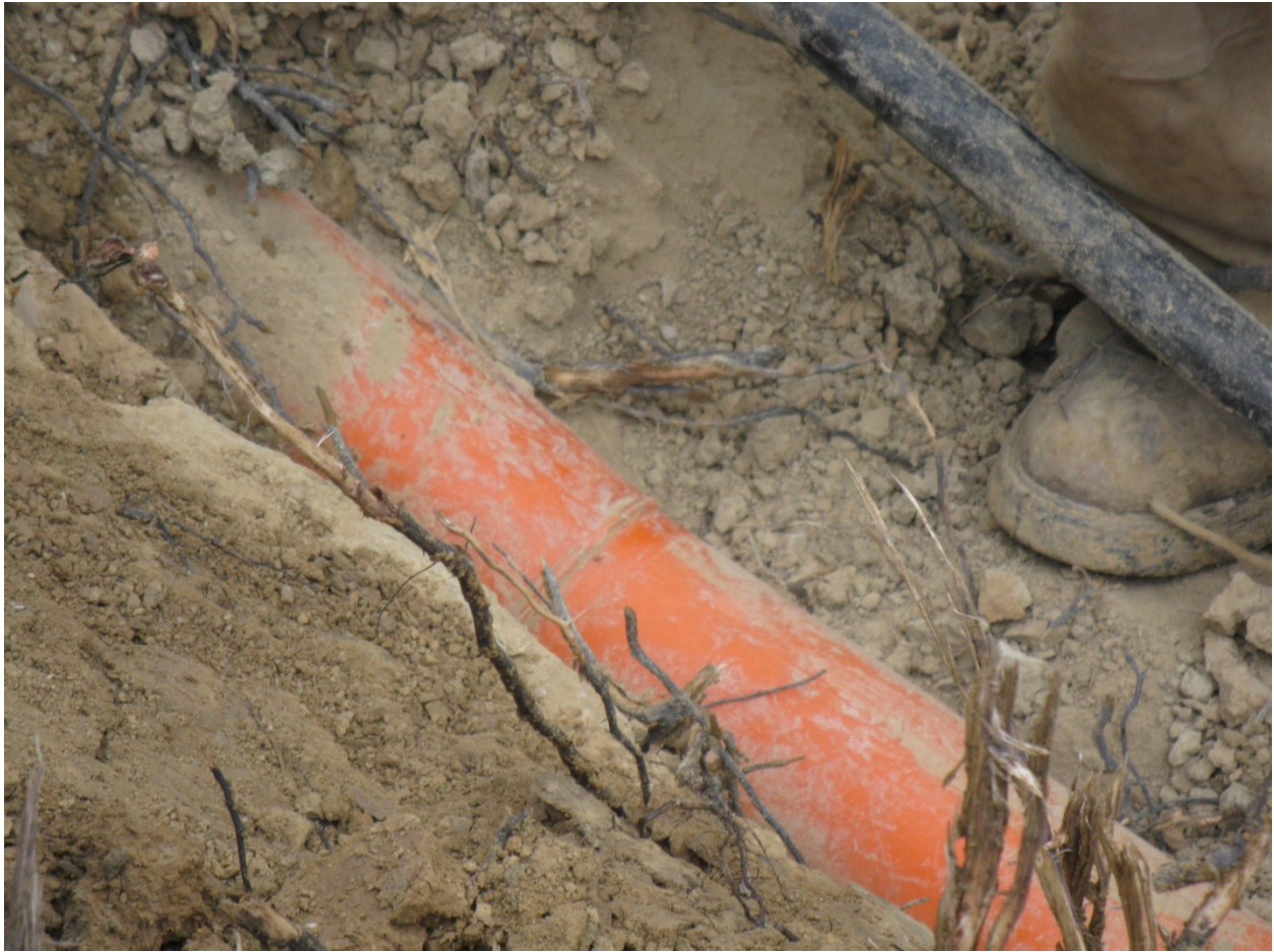
Photograph # 18 – 5730 Mango Drive, looking down at the leak location on the main. Note the dry soil around the leak location (Photograph taken by Staff).
