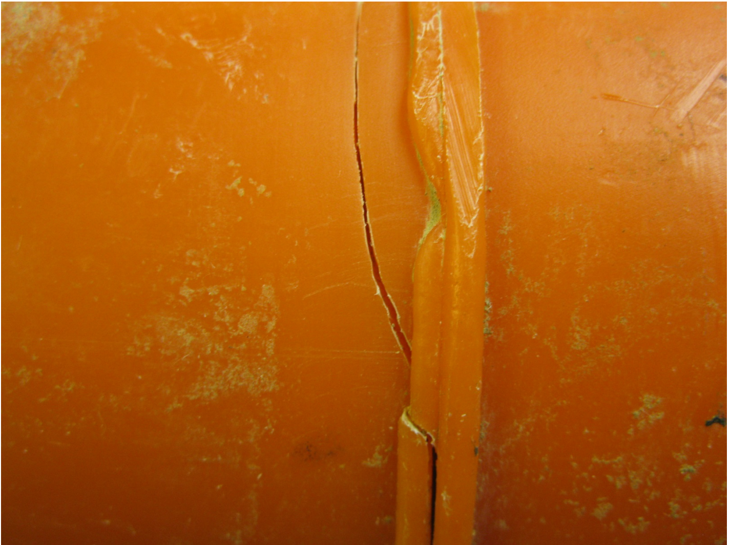
Photograph #1 –Failed Butt heat-fusion joint showing void in fusion bead (upper part of photo) and failure in the fusion joint (lower part of photograph). The failure in the fusion joint indicates that the joint was not stronger than the body of the pipe at this location. (Photograph taken by Staff, September 12, 2016).
