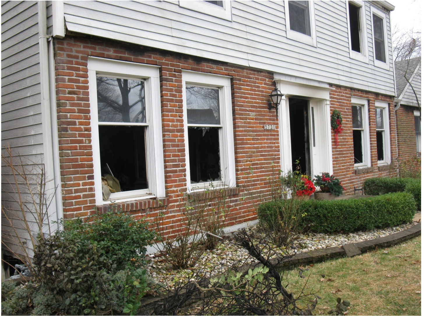
Photograph #13 - Front Side of 5730 Mango Drive, showing damage at front of house (Photograph taken by Staff).
