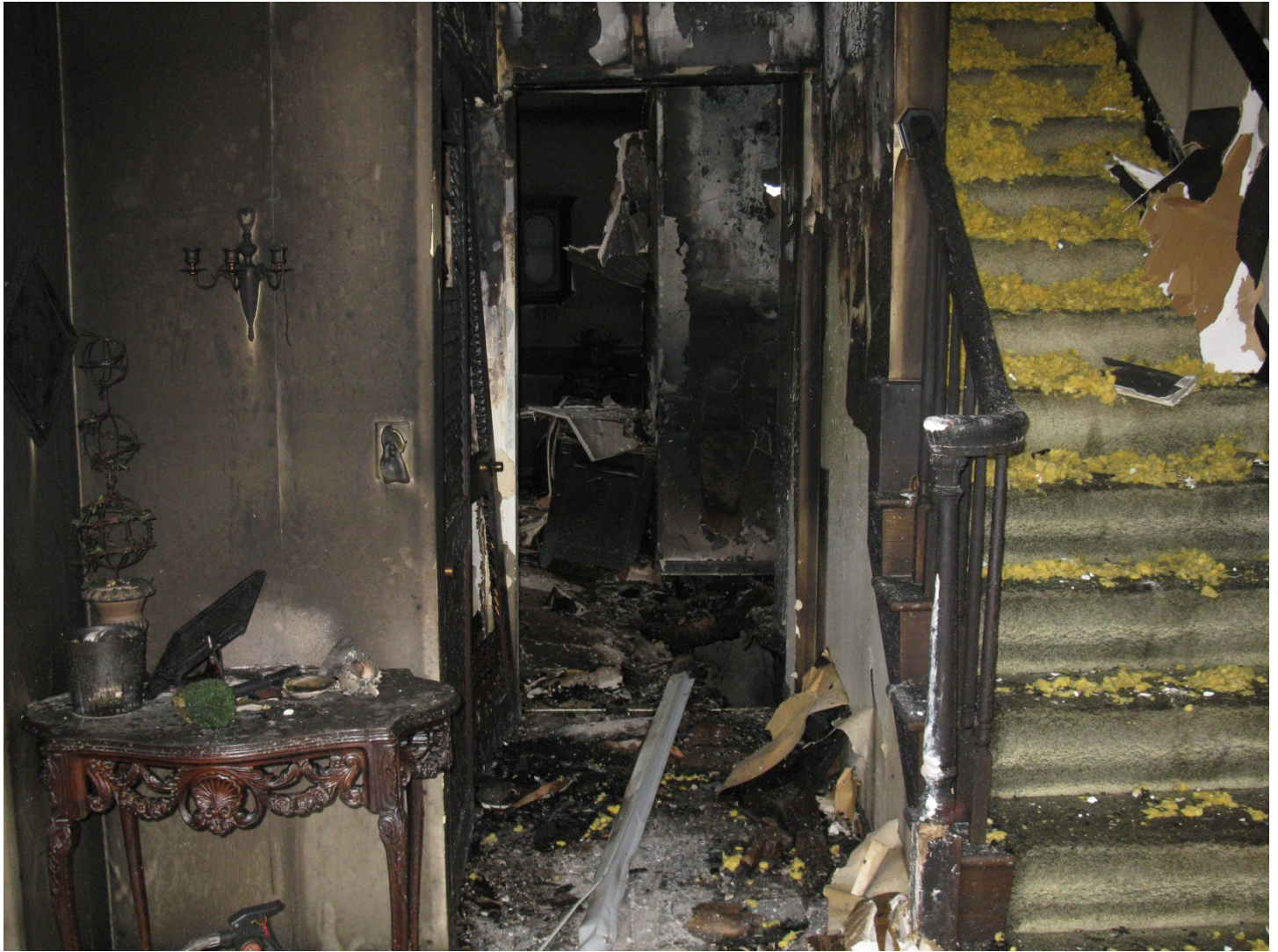
Photograph #16—Showing damage inside at front entrance to 5730 Mango Drive (Photograph taken by Staff).
