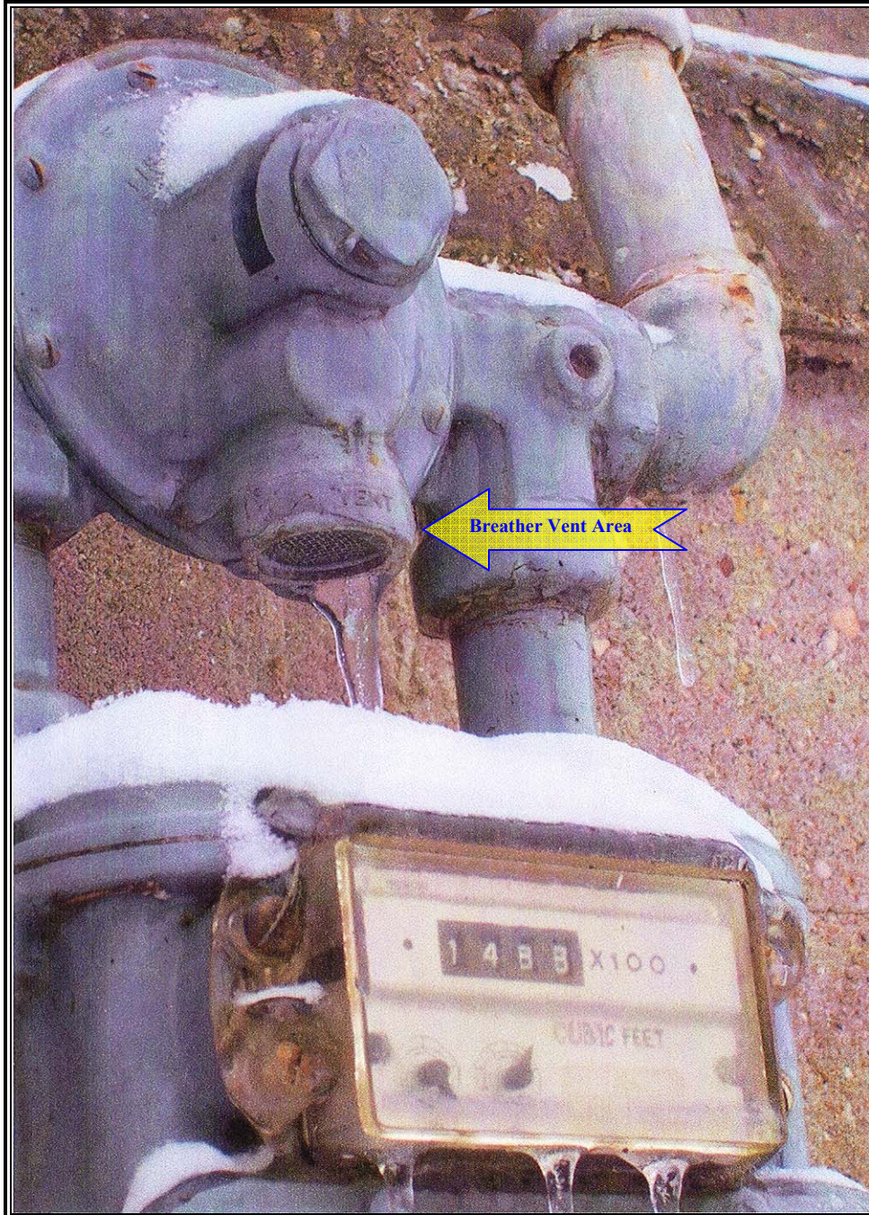
Photograph 7 Close-up view of the natural gas meter set for 715 E. 4 th Street in Milan. This picture was taken by WCE personnel on January 8, 2005 after learning that the house fire may have involved natural gas. Observe the icicles hanging from the breather vent area of the regulator and the meter index cover. On this date, WCE personnel verified that the regulator vent screen (breather vent) had been iced over and blocked.
