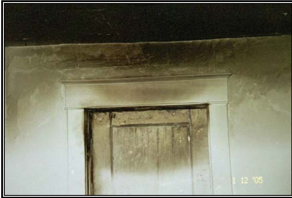
Photograph 3 View looking north (from the dining room) at the south door for the bathroom area. This door was closed at the time of the natural gas incident. The top portion of the door received heat and smoke related damage. The dining room received smoke related damage.
