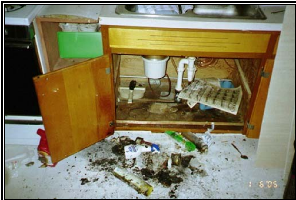
Photograph 8 Looking at the area beneath the kitchen sink. A light blue plastic tub can be seen covered by newspapers (to the right of the P-trap). The kitchen cleaning items on the floor were inside of the light blue plastic tub, but were later removed by fire department personnel in order to extinguish the fire. This was the only indication of fire damage on the main level. The gas range can be seen to the left of the kitchen sink.
