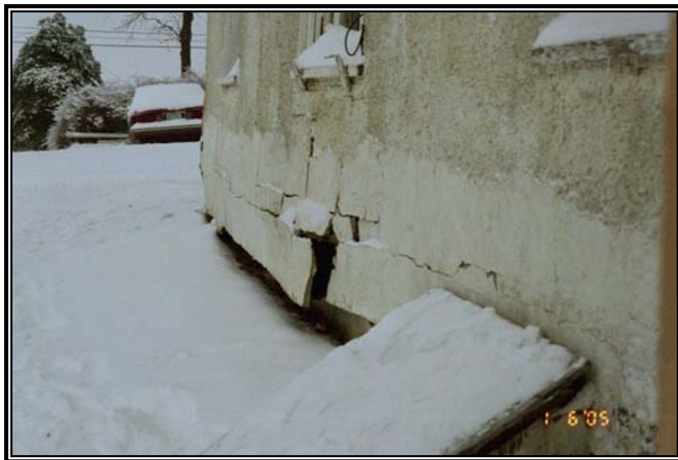
Photograph 4 Close-up view of the damage to the exterior west wall. Note how the wall was buckled and displaced outwards from the foundation. The greatest damage to the west wall was observed from approximately the basement entrance to the northwest corner of the building. The basement access cover was placed over the entrance just prior to taking this photograph.
