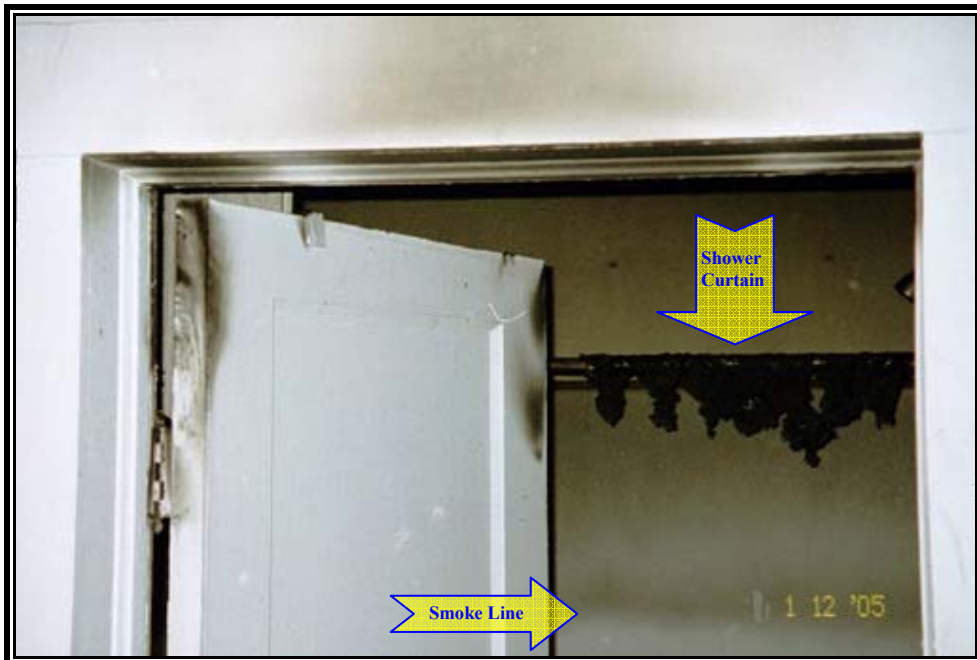
Photograph 4 Looking to the east at the bathroom area that received the most severe fire and smoke related damage in the home. This photograph was taken from the kitchen area of the residence. This west door to the bathroom was also closed at the time of the natural gas incident.
