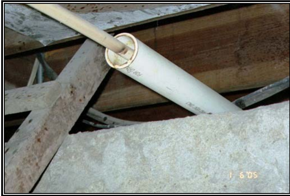
Photograph 7 View of the PVC water line that traversed east from the outlet side (hot) of the water heater to the kitchen sink that was also located east of the living room. The larger diameter PVC pipe was used as a conduit to protect the water line. Observe the light brown discoloration of the PVC water line as it entered into the PVC conduit.
