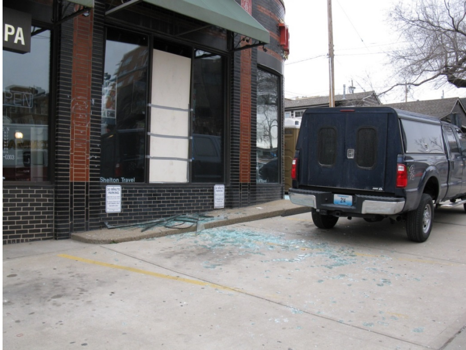
Photograph #13 – Damage to various businesses in the strip mall located southeast of the intersection of W. 48 th Street and Bellevue Avenue. (Staff Photo)
