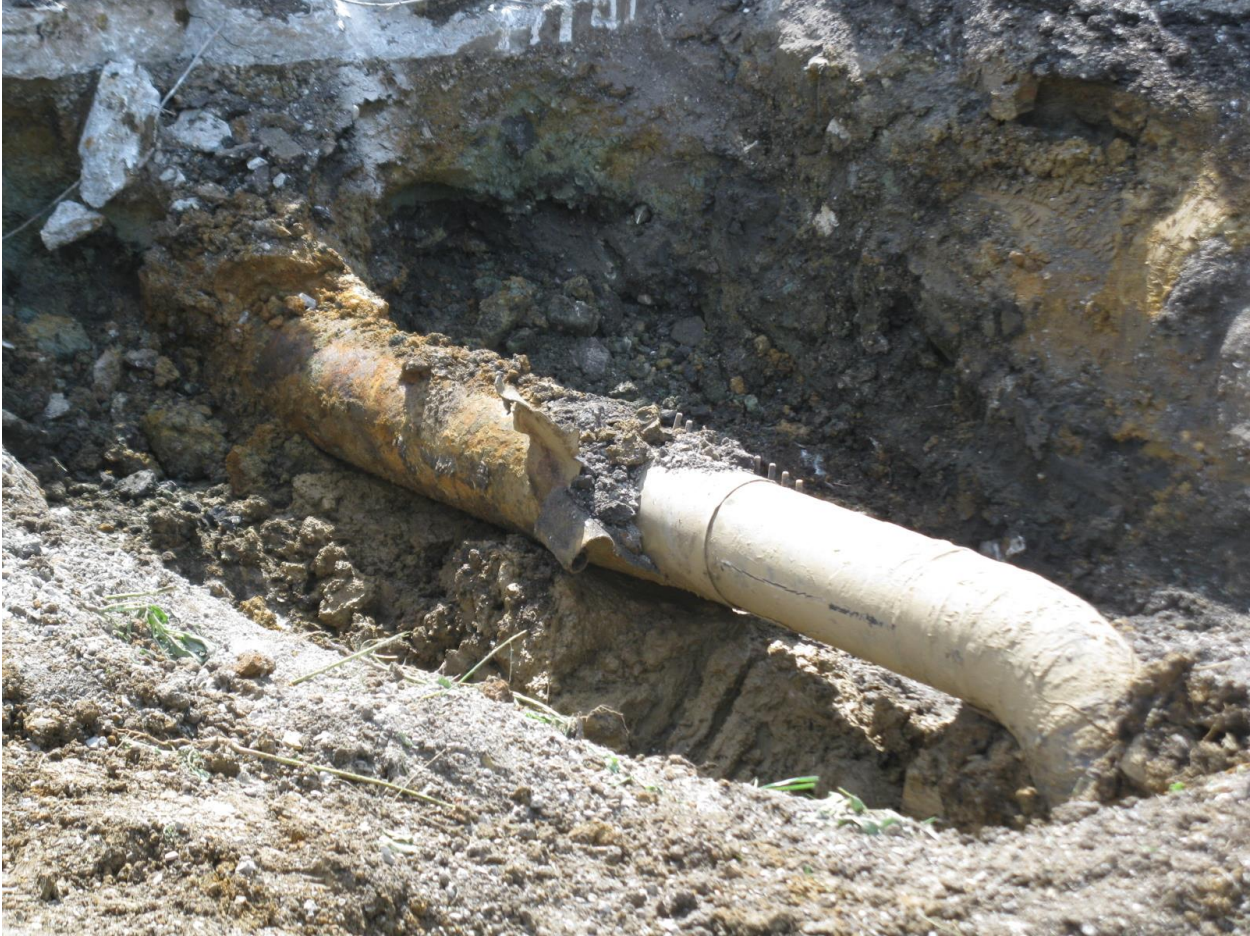
Photograph 4: Photograph of the damaged portion of the pipeline looking southeast. A repair clamp is surrounding the damaged portion of the pipeline. (Source: Staff)
