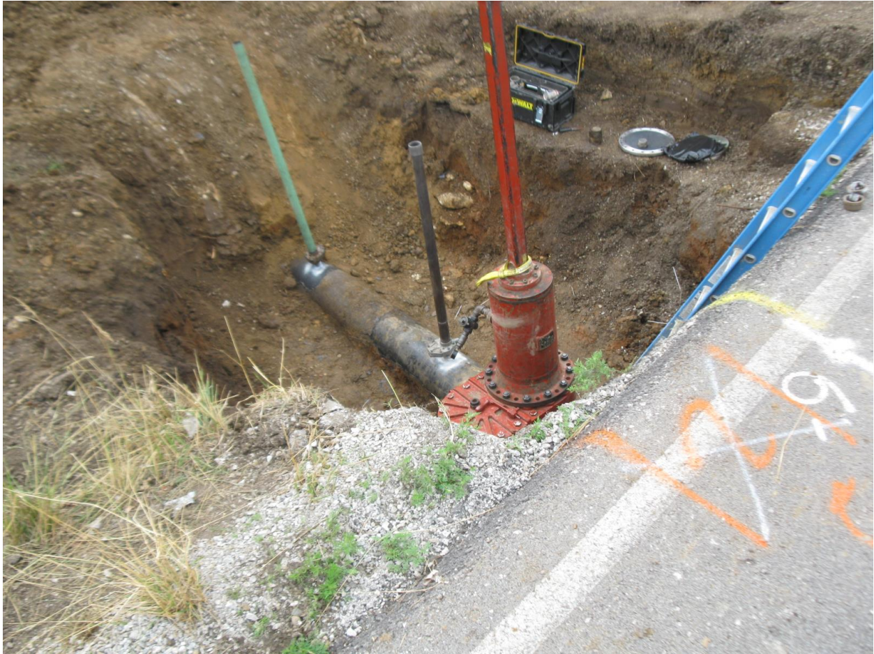
Photograph 2: Photograph of tapping and line stop fitting affixed to the pipeline on the west side of U.S. Route 169. (Source: Staff)
