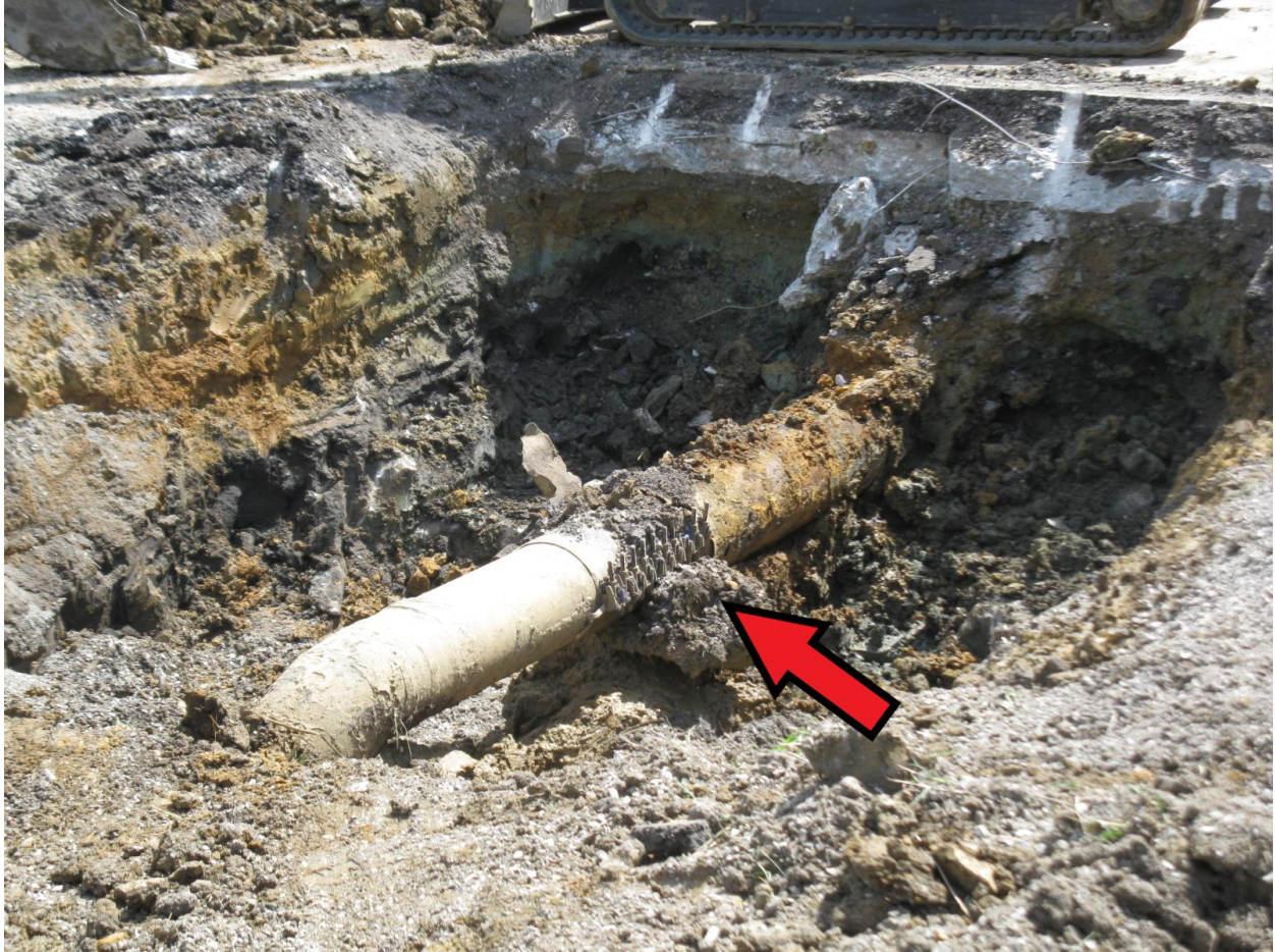
Photograph 3: Photograph of the damaged section of pipeline looking northeast. The red arrow (added by Staff) points to a repair clamp surrounding the damaged portion of the pipeline. (Source: Staff)
