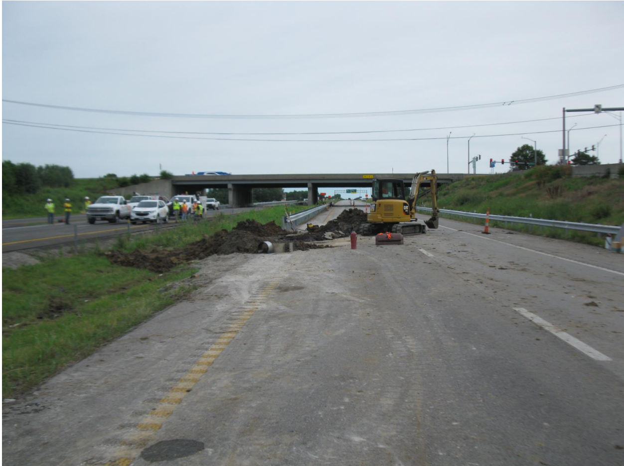
Photograph 1: Photograph looking north along the northbound lanes of U.S. Route 169 toward Northwest Barry Road overpass. The excavation in the median contains the damaged pipeline. (Source: Staff)
