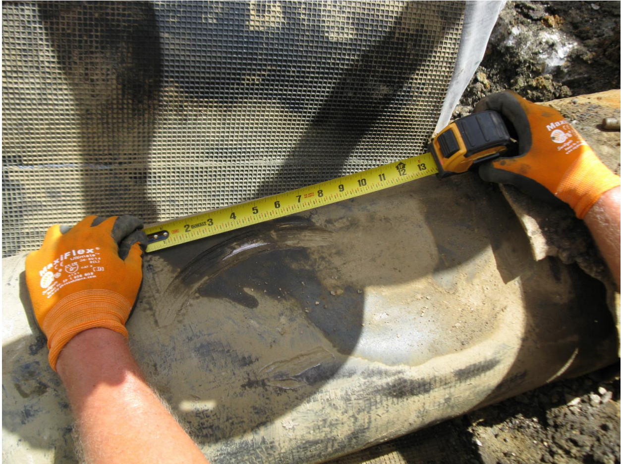
Photograph 5: Photograph of the damage to the pipeline. (Source: Staff)
