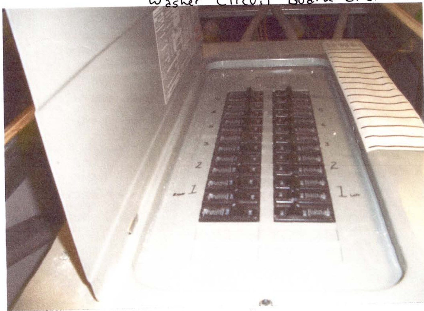
Washer Breaker Box
