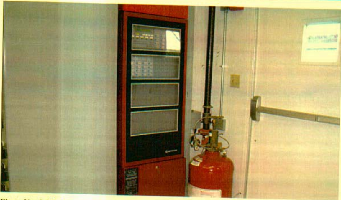
Photo No. 2.6-1 - Fire Suppression System Control Panel, located in Electrical Package.
