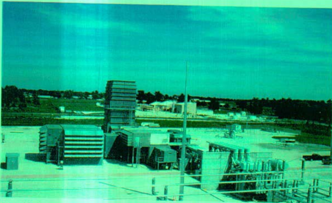
Photo No. 2.1-3 – Units 3 and SS Compressor Station
