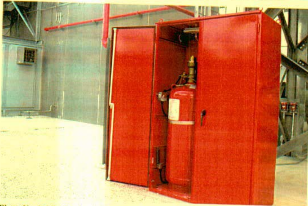
Photo No. 2.6-3 - Combustion Turbine Enclosure with FM-200 Bottle.
