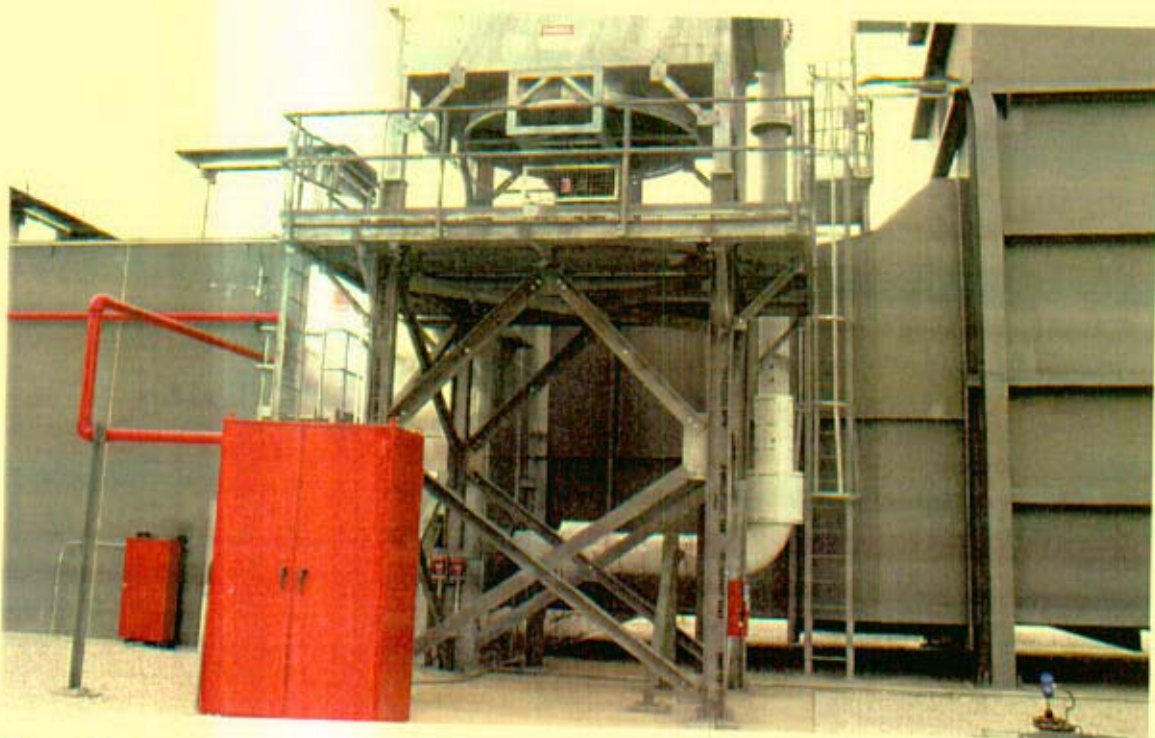
Photo No. 2.6-2 - Combustion Turbine Enclosure FM-200 Cabinet
