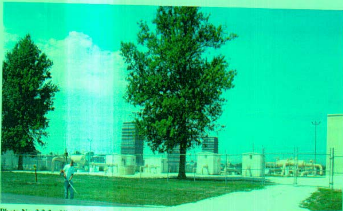
Photo No. 2.2-2 – View looking west to southwest from the corner of South Harper Road and 243rd Street (foreground is the existing Southern Star Gas Compressor Station).
