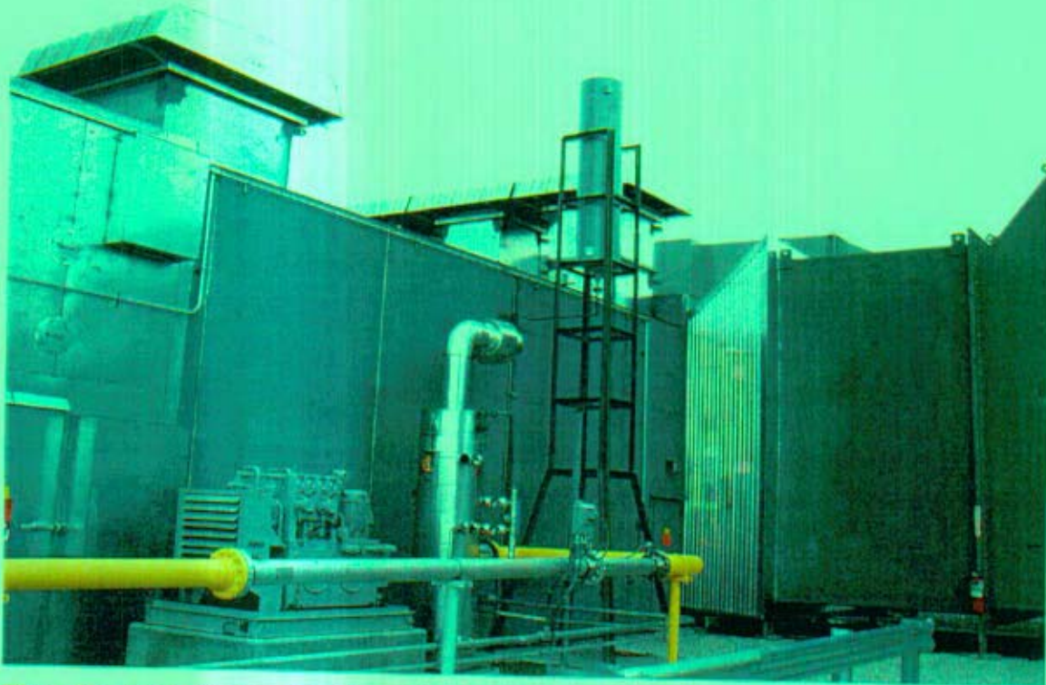
Photo No. 4.2-2 – Turbine Gas Vent Silencer
