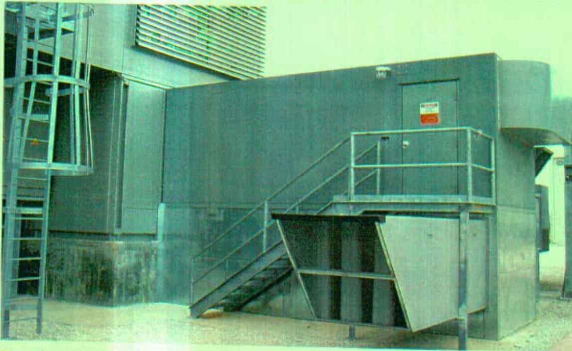
Photo No. 4.2-5 – Starting motor package ventilation silencer
