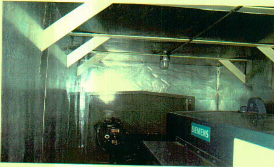
Photo No. 4.2-8 – Starter motor enclosure (internal)
