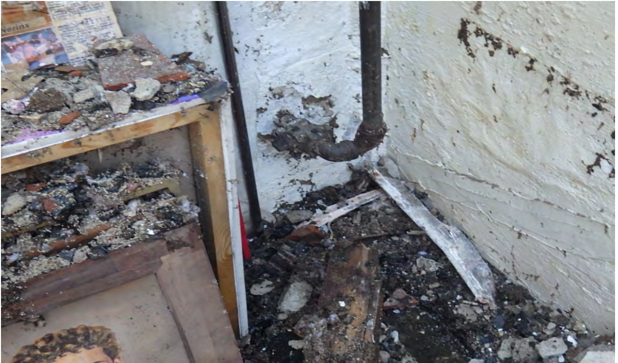
Figure 10 – Service Line In Basement
