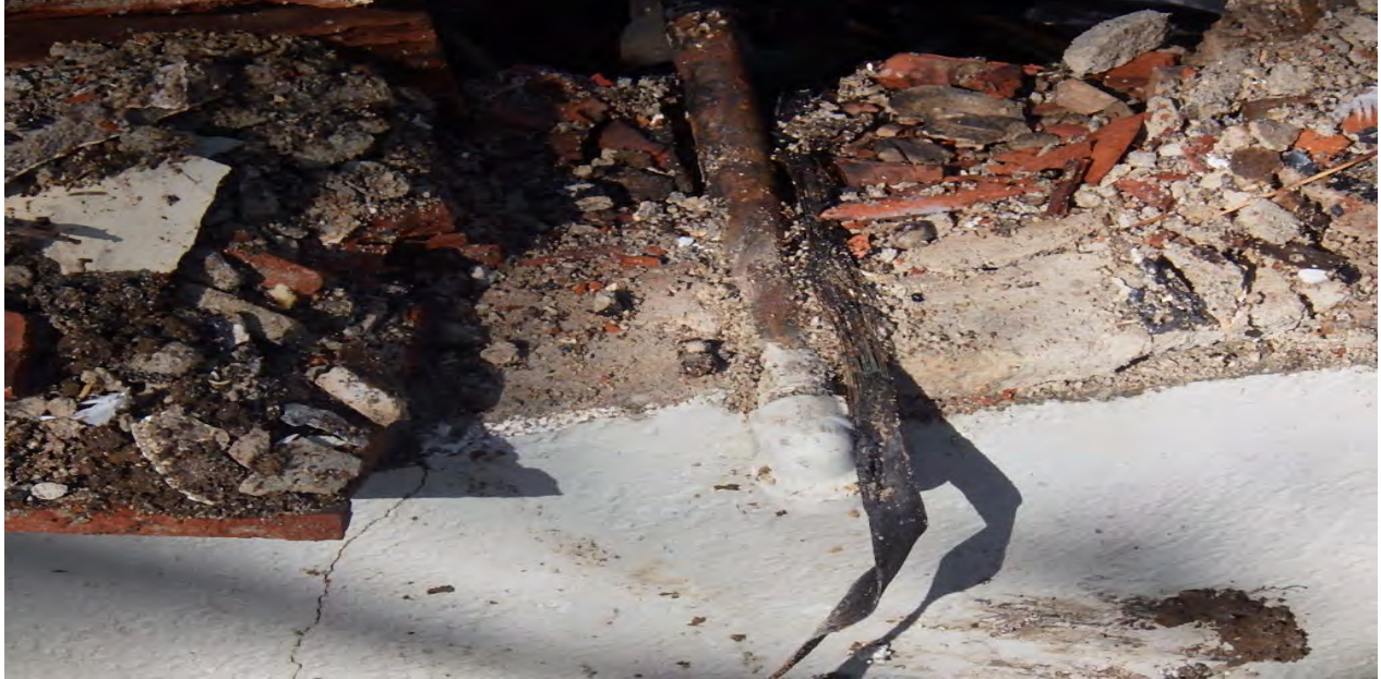
Figure 7 – Inside Meter Vent
