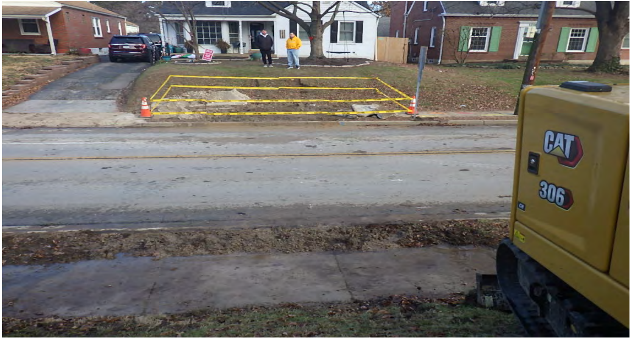
Figure 5 – Location of Spire Excavation Made in Attempt to Find Gas Curb Valve
